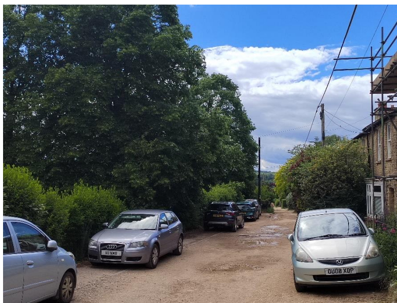
Potholes in Charlbury
